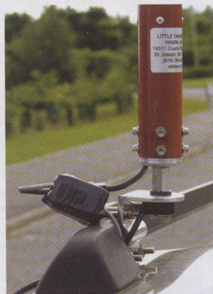
The antenna requires a meaningful mounting bracket. The control cable ferrite core (foreground, left) is wrapped in insulating tape.
